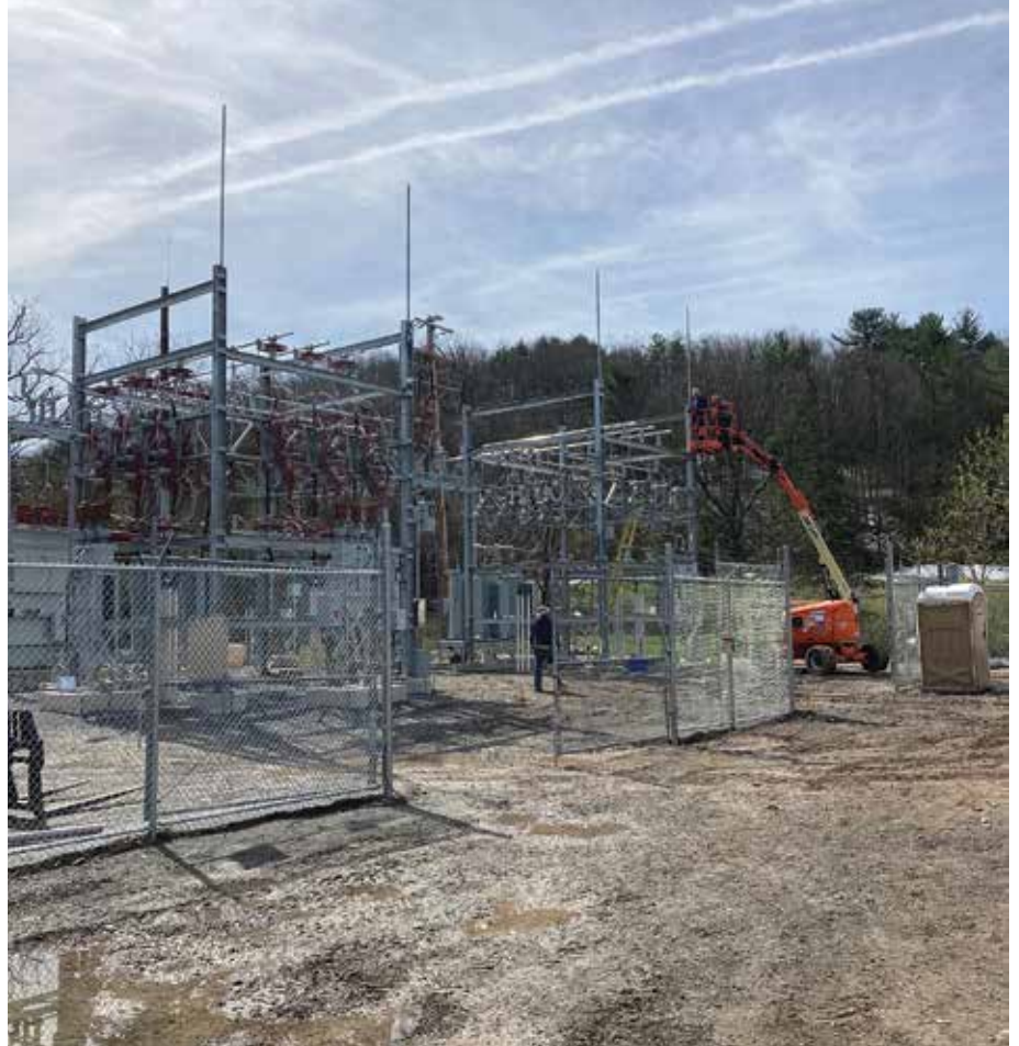
ALMOST THERE: Construction nears completion at the new Waterfall substation, which is a welcome addition to the cooperative's plant.
