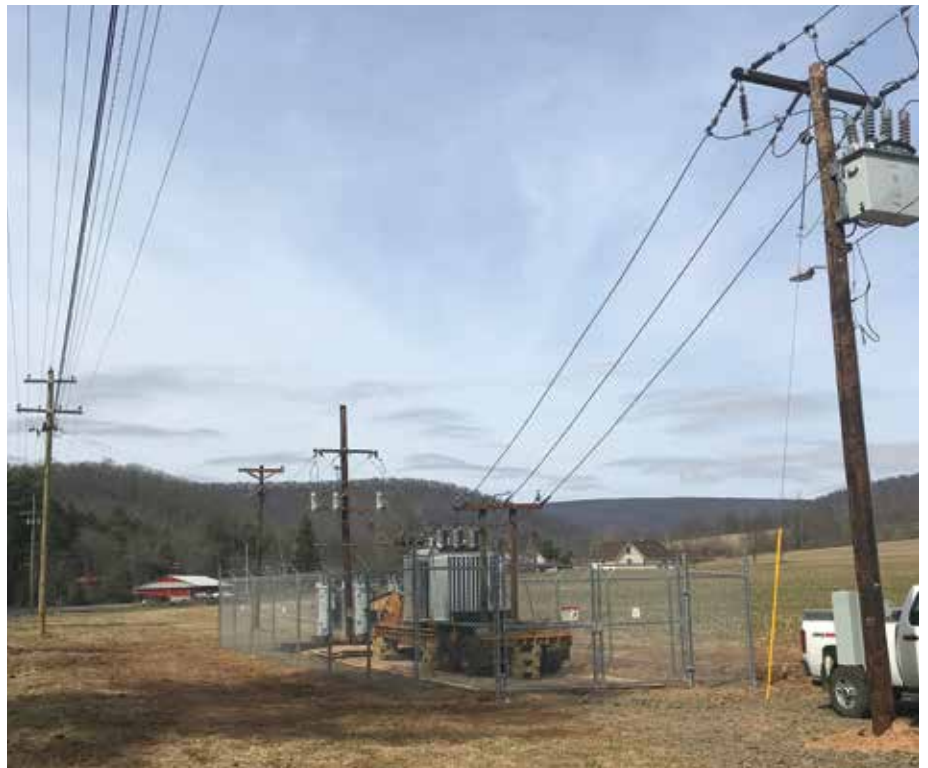
WORKING SMARTER: A temporary substation was brought online during the Waterfall project to increase safety and efficiency.
