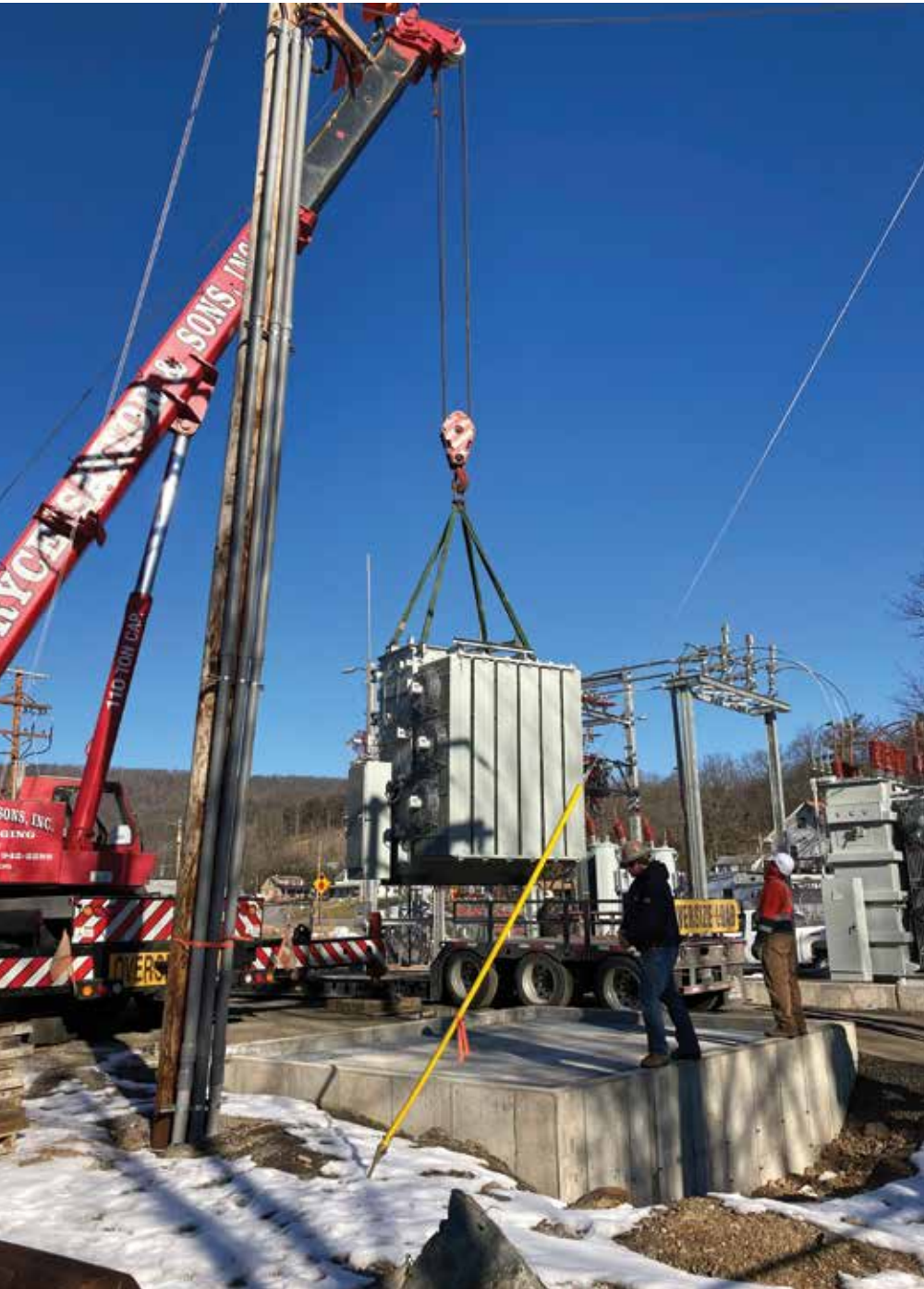
TRANSFORMER ARRIVES: Crews direct the placement of the Bay 2 transformer at the site of the new Waterfall substation.
